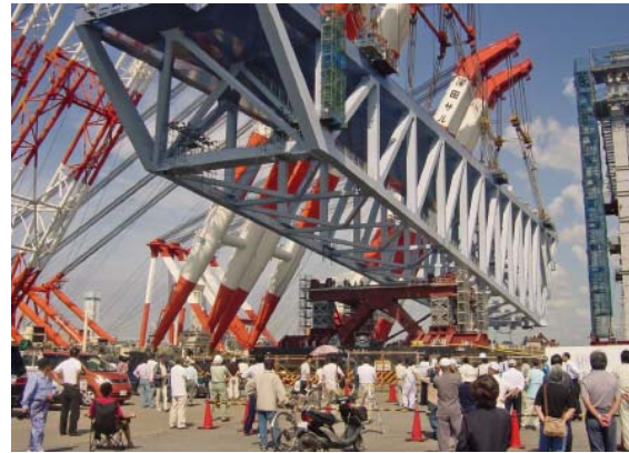
▲ Launching the truss girder off the fabrication yard (Futtsu City, Chiba Prefecture)
