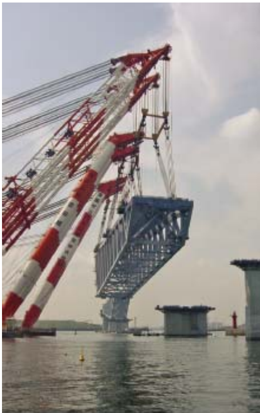
▲ Hoisting the truss girder on the Wakasu side, at two lift points each, using three floating cranes
