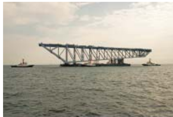
▲ Towing the truss girder on a barge type platform (capacity: 24,000 tons) to the erection site
