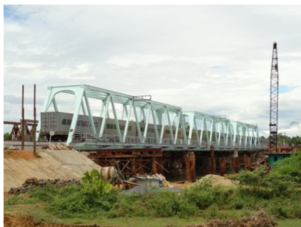
CP1D construction zone - Tien An Bridge (Quang Tri) Tekken Corp., Yokogawa Bridge Corp., Thang Long Construction Corp. JV
