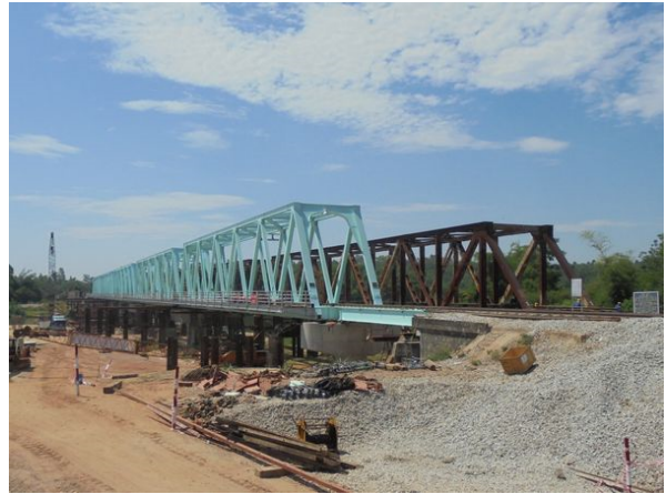
CP3A construction zone - Tra Bong Bridge (Quang Ngai) Tekken Corp., Mitsui Engineering & Shipbuilding, Thang Long Construction Corp. JV
