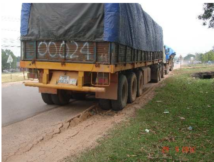
Damage to old paving as a result of use by excessively heavy vehicles (vehicles from Vietnam)
