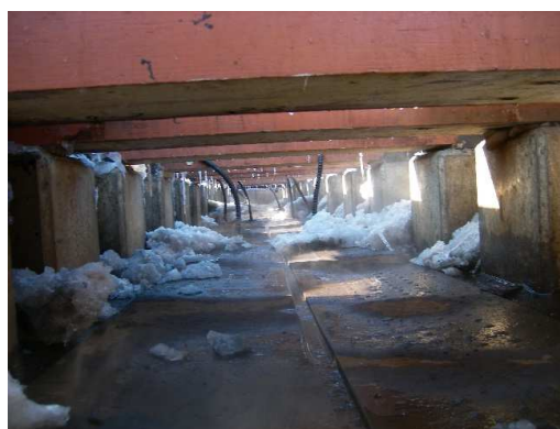
View of Inside Switch Snow-Melting Pit
