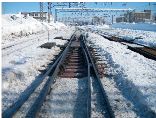
Switch Snow-Melting Pit (Installed on the Hakodate Line at Iwamizawa Station)
