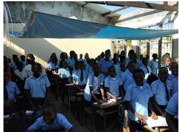
Macurungo Elementary School Roofs were blown off by Cyclone Idai, May 2019.
