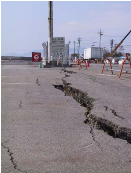
Cracks on a Wharf at Kusatsu Area, Hiroshima Port
