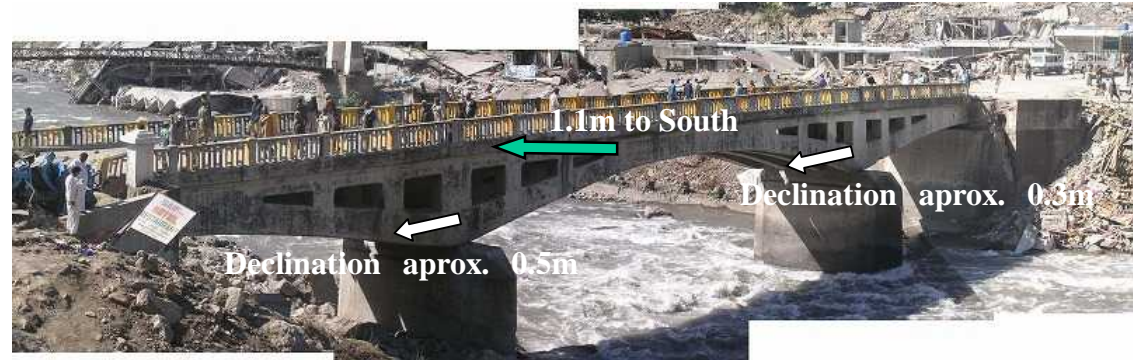
Displaced Bridge Girder due to Earthquake Motion(Pakistan)
