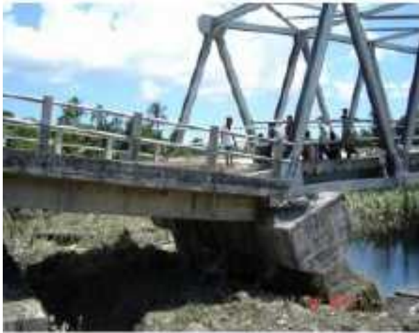
Tilted and Sunk Pier of Bridge due to Liquefaction(Indonesia)
