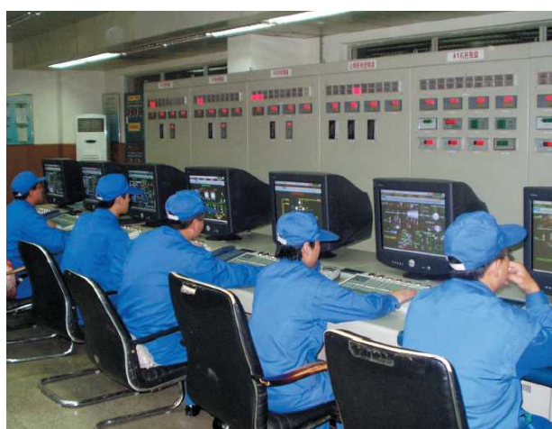
Photo 9 Central control center of the plant. Plant operators are receiving training during the construction stage of the plant.
